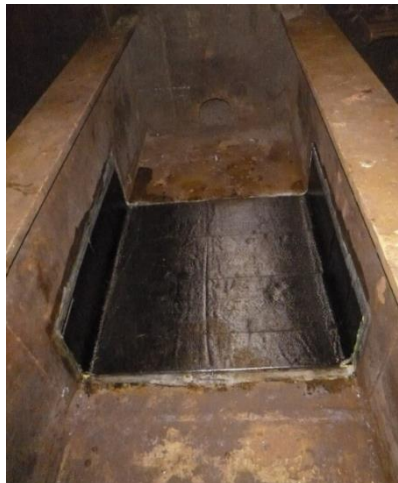
Figure 1. Structural composite repair on ship bottom plate using Carbon Fibre Reinforced Polymer (CFRP) [11]
